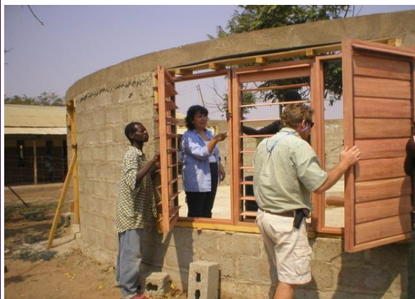
Photos taken at the construction site in September, 2006, show the walls, floor and windows of the first Lubuto Library, at the Fountain of Hope in Lusaka, Zambia, beginning to take shape. (from http://www.lubuto.org/ )
